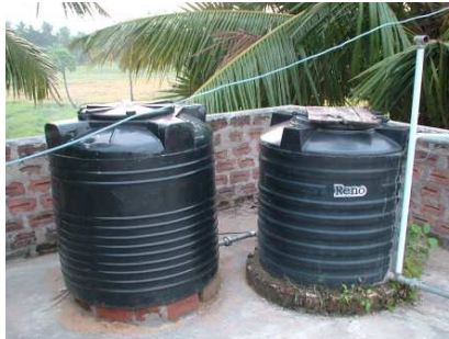
Left: Job done! The new water tank, on the left, in place and linked with the old tank.
